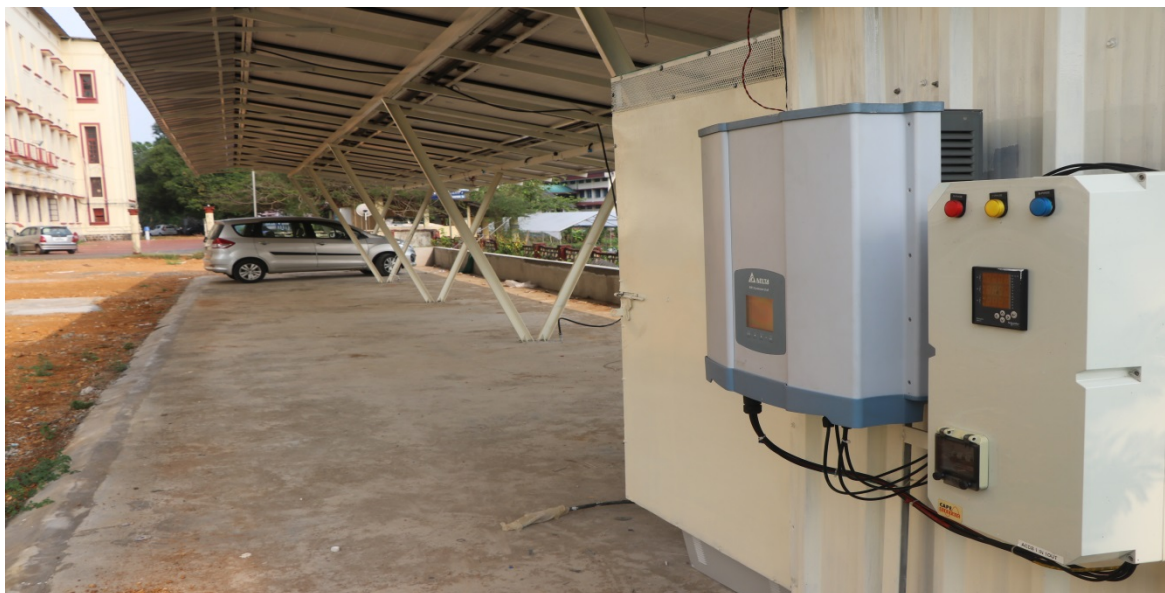
Solar Energy Harvesting Plant
